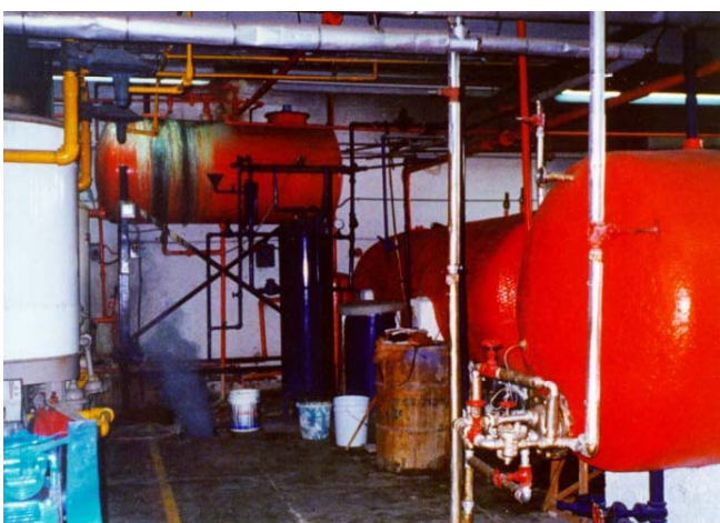
Old Steam Generators and Hot Water Tanks
