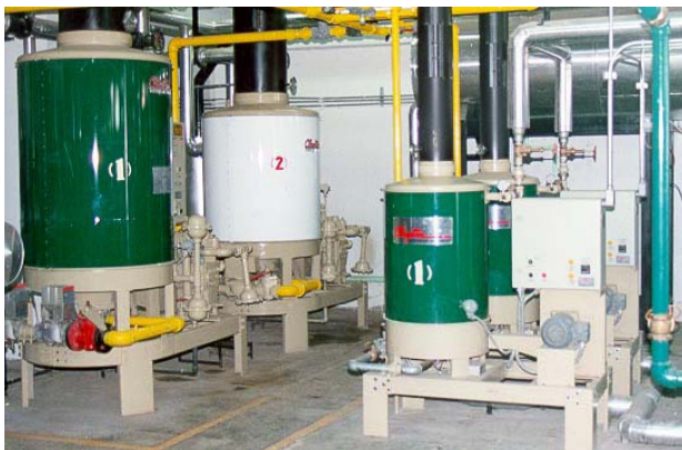
New Presence of the boiler room
