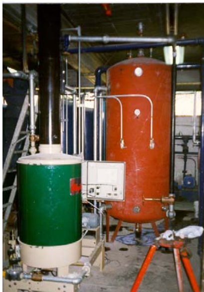
Small tank for direct hot water recirculation
